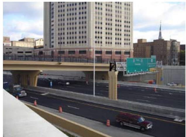
Work on the North Leg portion of the Marquette Interchange Project is virtually complete. The North Leg achieved a 25.8% DBE share through November 30, 2006.
